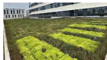
Rooftop Greening in Ningbo Factory
